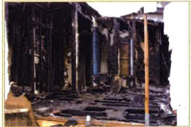
The back half of a residence on Herald Road sits gutted after a fire ravaged the back of the house.
